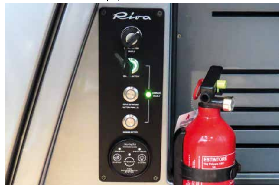
Fire extinguisher control panel
