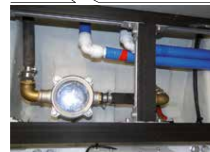
Air conditioning unit sea cock
