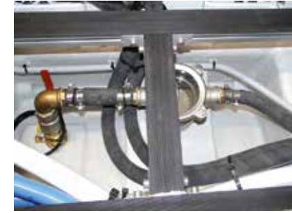
Generator sea cock
