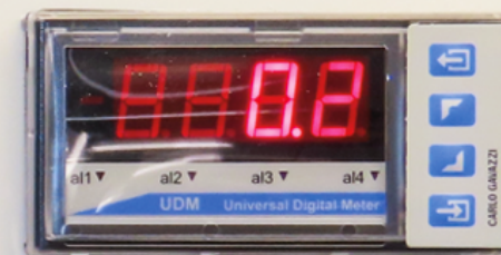
ENGINES BATTERY VOLTAGE
