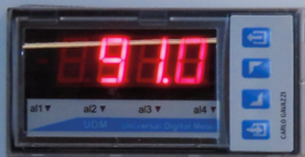
SERVICE BATTERY DISCHARGE CURRENT
