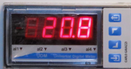
ENGINES ROOM AIR TEMPERATURE
