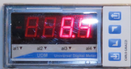
SERVICE BATTERY VOLTAGE
