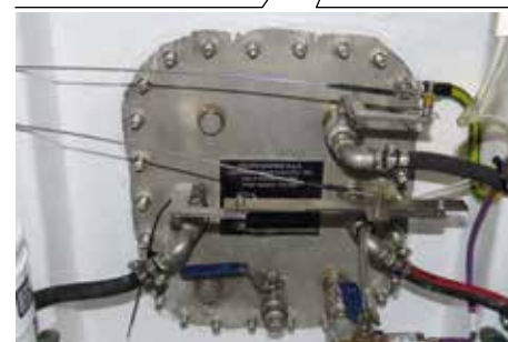
Fuel distribution valves
