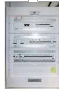
Engine room electrical panel
