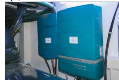
Service battery charger and inverter (optional)
