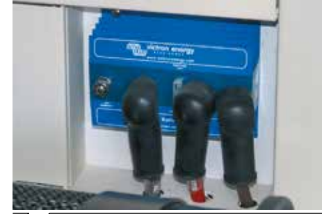
Engines battery charger
