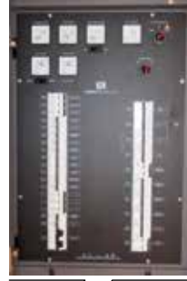
Main deck electrical panel
